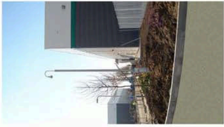
EXISTING CCTV COLUMNS AND CCTV CAMERAS
